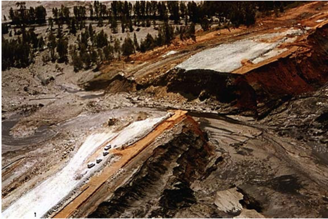
Figure 3.5. Breach of the broken tailings pond dam (from Aguilar et al. 2000)
