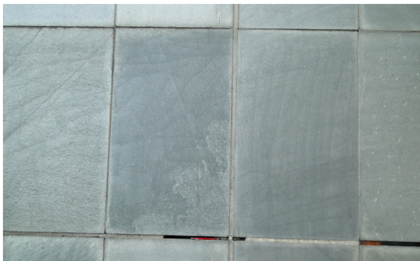
Figure 8. Phyllitic Quartzite facade panels (transverse length = 50 cm) (almost 60 years old); Alta Quartzite/Norway.
