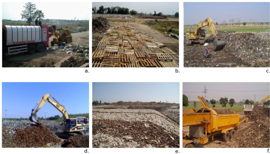
Figure 4.12: Mechanical and biological treatment of Thailand: a) waste is put inside the mobile rotary drum to open closed plastic bags; b) wooden pallets and slot pipes are placed on the ground of landfill; c) the windrows of waste are constructed by an excavator; d) constructed windrows are covered with coconut husks as bio-filters; e) non turning windrows for 9 months; f) after 9 months, material is sieved for further utilization
